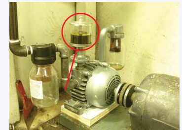
Vacuum Pump is beneath breaker panel. Verify clean oil is in top reservoir. If not "do not use". Notify staff.
