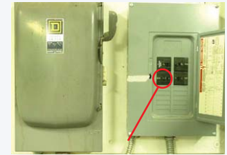
Breaker panel to turn on Vacuum pump. Lower left breaker marked with tape. Panel located behind machine.
