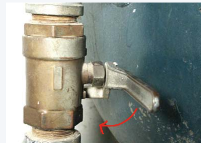
Reserve tank valve. Shown closed, push down to open.
